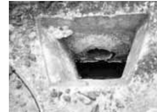
In this picture, looking down an outlet baffle, the effluent is below the pipe, indicating a bad seal.
