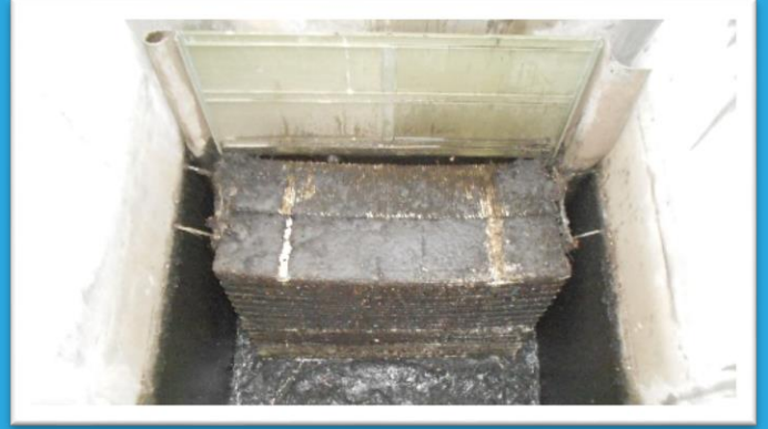
Oil/Water Separator before cleaned
